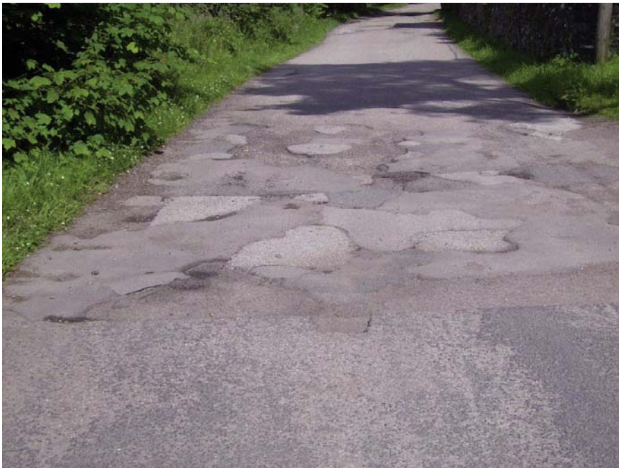
Rural road that has been continually potholed and verges very overgrown.
